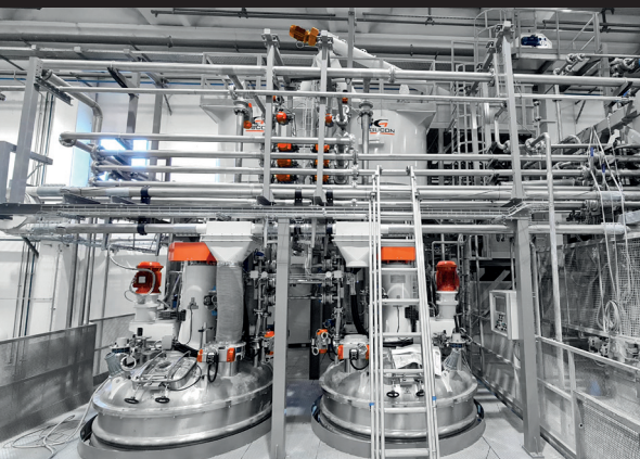
Impianto completo pitture Complete paint production plant
